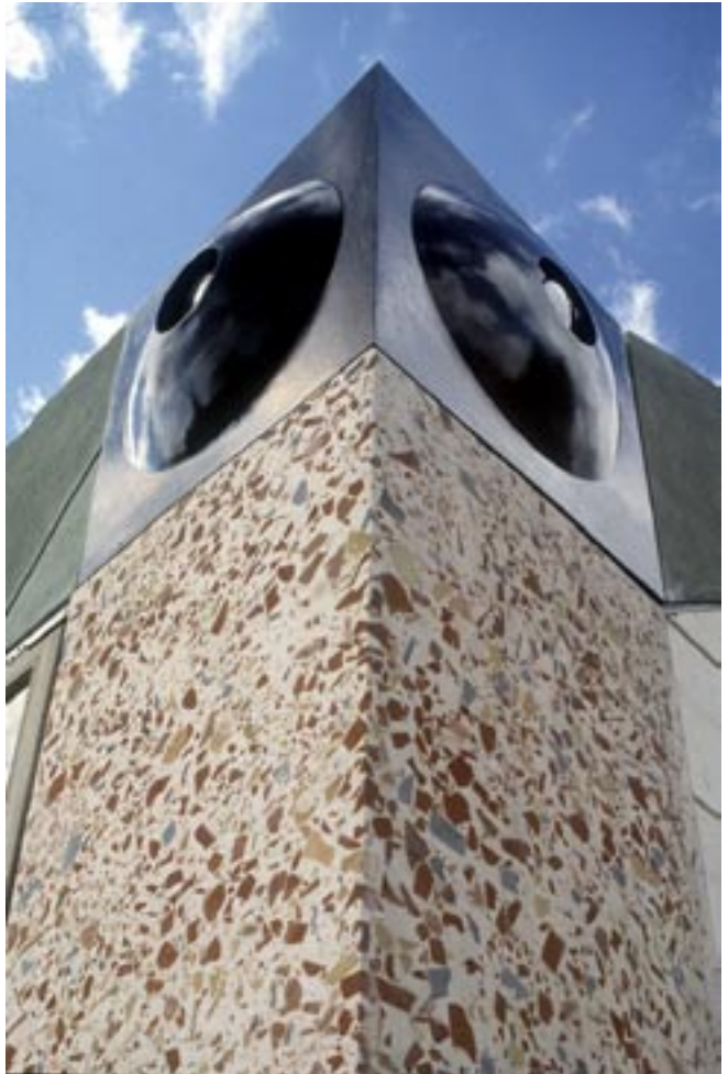
The first use, back in 1981, of 150mm (6") thick 'Blitzcrete' concrete that was made from five different brick types. The bricks were washed, after breaking, to remove dust that would colour the silver sand and white cement background. Stainless reinforcement was held in the grey concrete backing layer. The corner was cast in two continuous pours. 5mm (1/4") is ground off the surface during the short time the concrete is 'green'.
